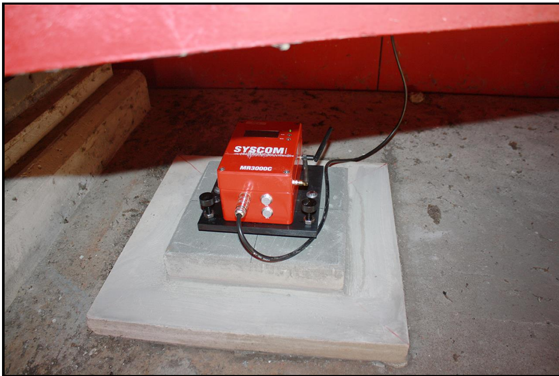
Figure 5 : Station de vibration
